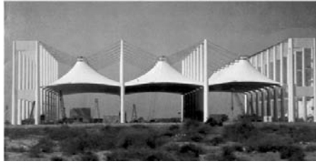
Figure 1-8 The Haj Terminal under construction, Jeddah, Saudi Arabia, 1981 (Photograph courtesy of Birdair, Inc.)
